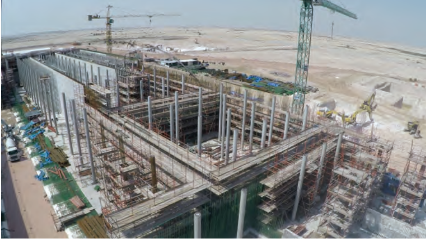
PLANNING Qatar is building five reservoirs to supply the country with seven days of drinking water.
